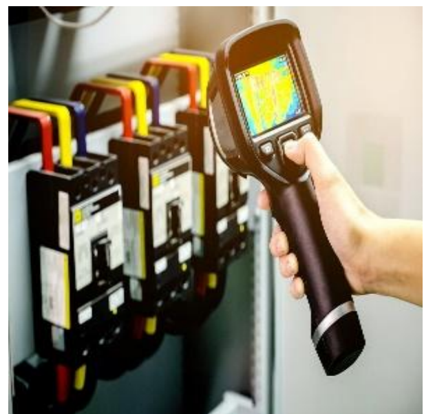
Figure 2: Thermograph on Electrical Panel
